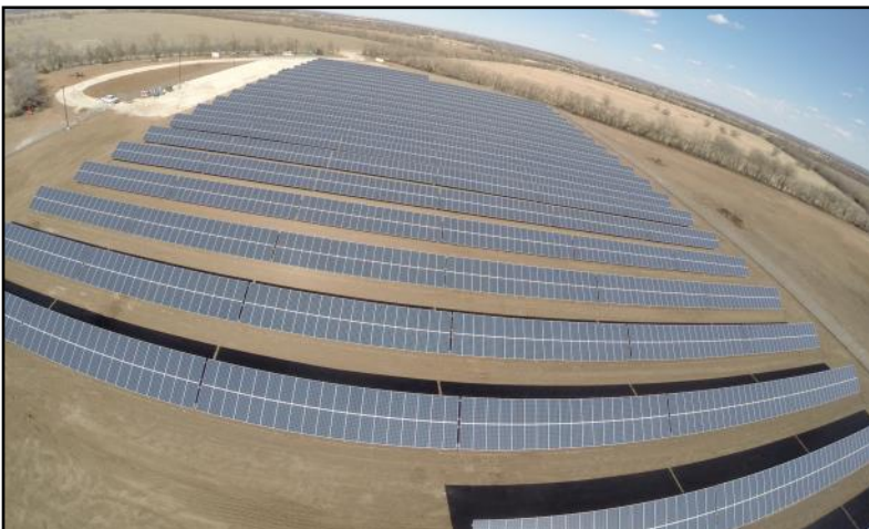
Prairie Sky Solar, a one MW solar facility located in Butler County.
